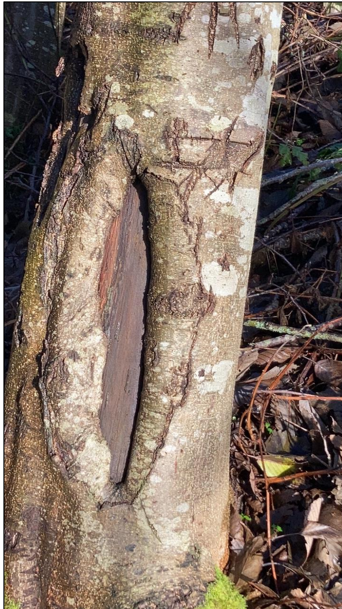
Photo 4: Tree 6604 with decay at base.
